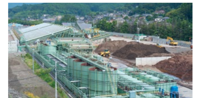
Salt removal equipment (Ofunato Plant) (as of 2012)
