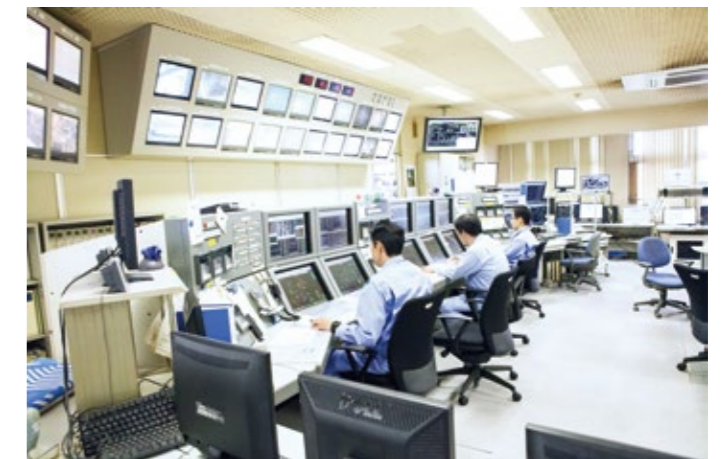
Central control room (Kamiiso Plant)
