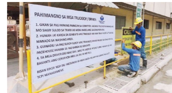
Posting of warning to drivers (Taiheiyu Cement Philippines, Inc.)
