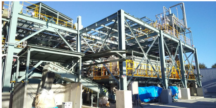
Photos of the demonstration plants; CO 2 capture facility (left) and carbonation equipment (externally heated rotary kiln, right).
