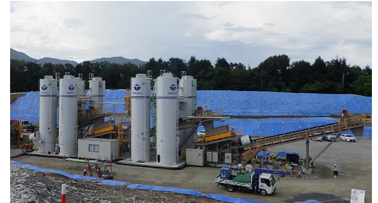
Multi-axial screening equipment integrated with crushing, classifying, and mixing
