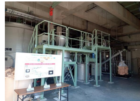
Phosphorus recovery and fertilizer conversion facility (B-DASH project)
