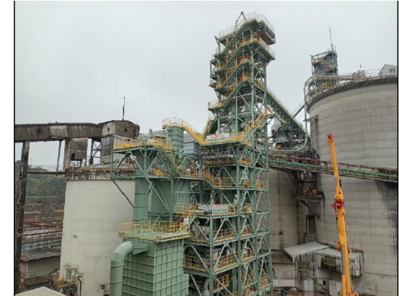
Saiki Ash Center, where classification facility is being installed (scheduled to be completed in June 2024)
