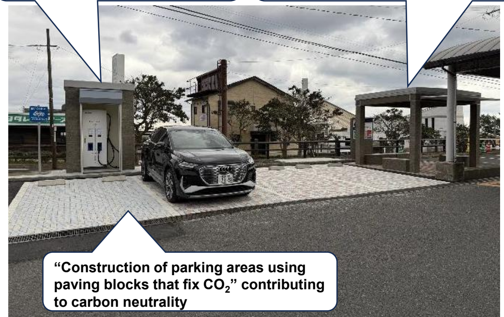
Installation of an EV quick charging station at “Life Center Yakuden,” a commercial facility located in Yakushima Town (example initiative)
