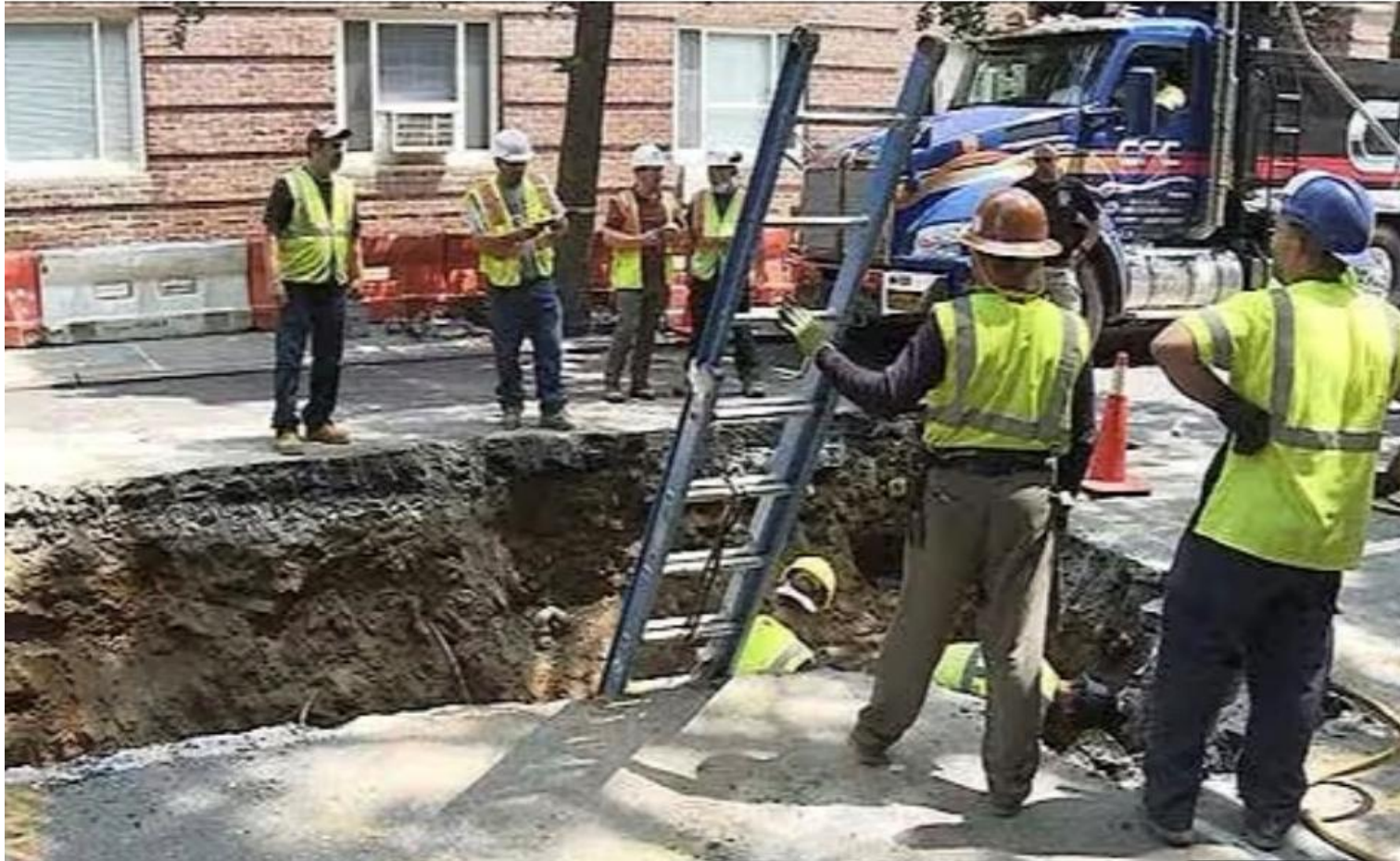
Road collapse in New York
